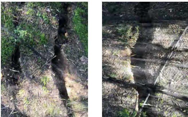
Figure. New erosion marks within the field area
