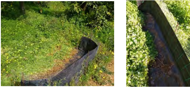
Figure. Orange orchard sediment fence (left) and Avocado trees sediment fence (right) after the 26/10/2017 rain event
